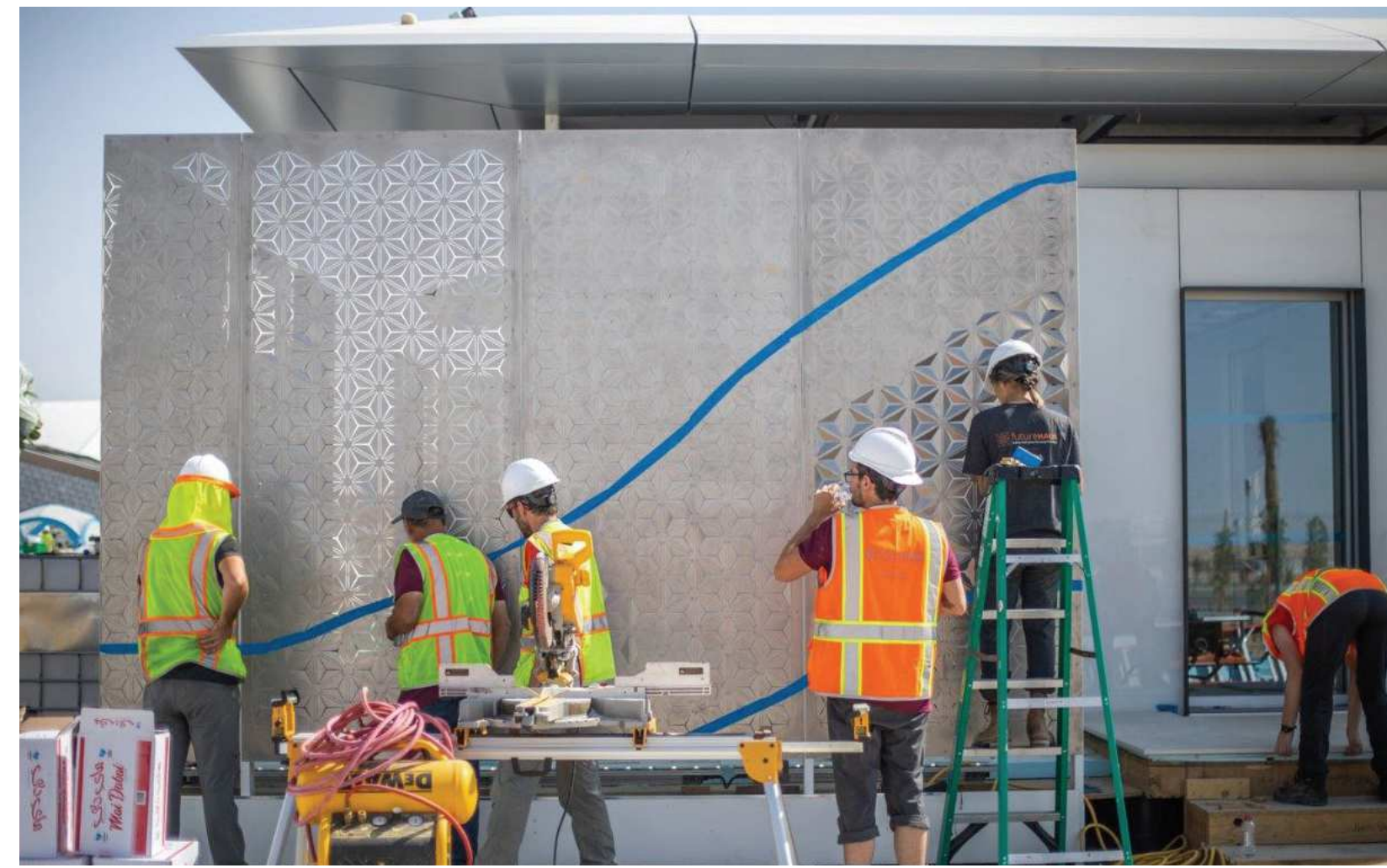
The flat screen wall is getting bent according to predetermined angles. (Photo by Erik Thorson Photography).
