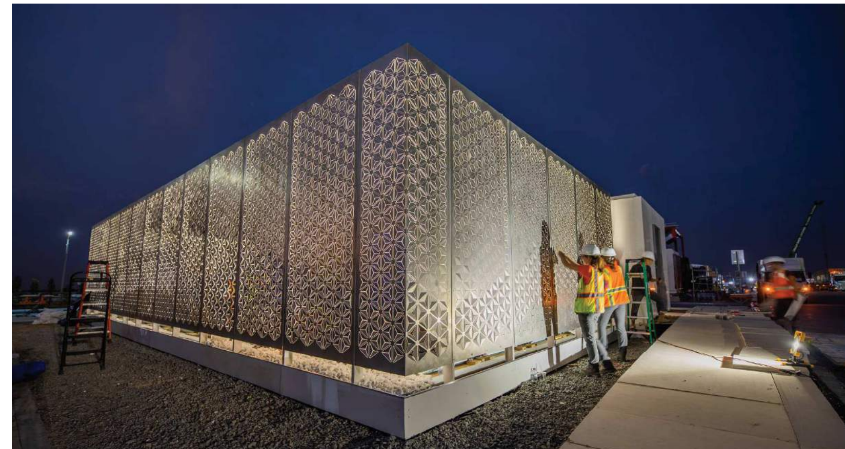
Small wooden jigs were produced for the crew on site to bend to exact angles. (Photo by Erik Thorson Photography).
